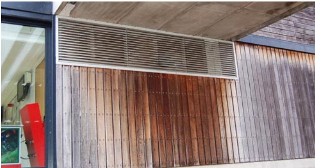
Figure 3 Typical shadow lines on cladding caused by differential weathering
