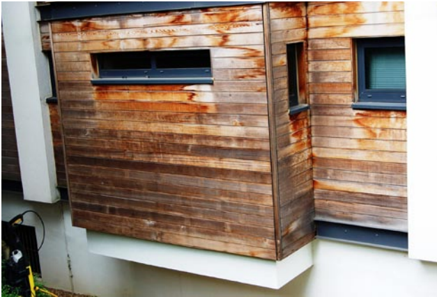
Figure 11 Discoloured western red cedar cladding before cleaning and treatment
